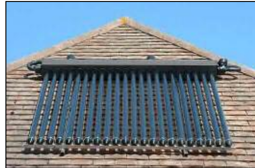
Solar Water Heating
